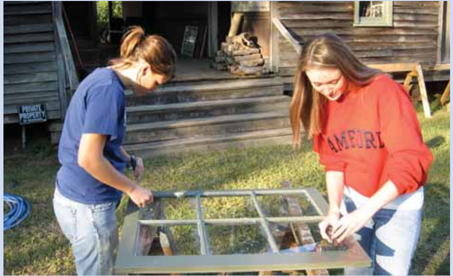
Students Kelly Fishbein, left, and Holly Morgan work on window repair at the 1836 Sadler Plantation Home in west Jefferson County.
